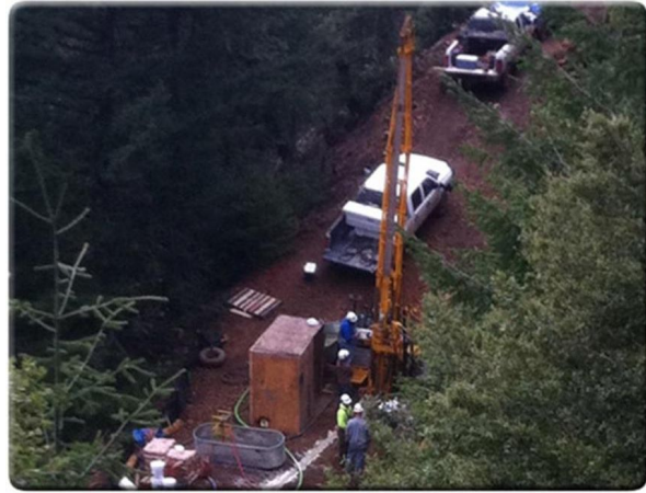
Fig. 22. Bore Hole Drilling at Turner Gold, (Reproduced from Josephine Mining Corp., July 2011, see Drilling at the Turner-Gold/Copper Property ).
